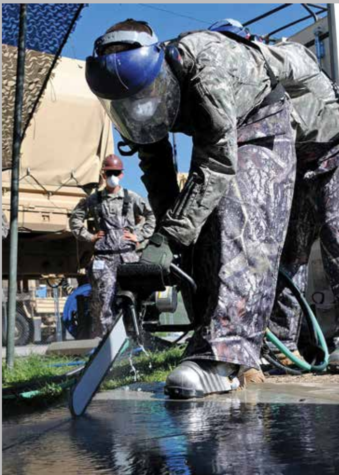
Spc. Kevin Gwilliam from the 624th Engineer Company, 1457 Engineer Battalion, uses a wet saw to cut a section of concrete as part of a renovation project on a restroom facility at the Renegade Point Marina, Strawberry Reservoir, June 8.
